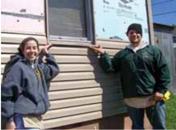
WVSOM Students installing siding on a home in Rainelle for 2009 Day of Caring.
